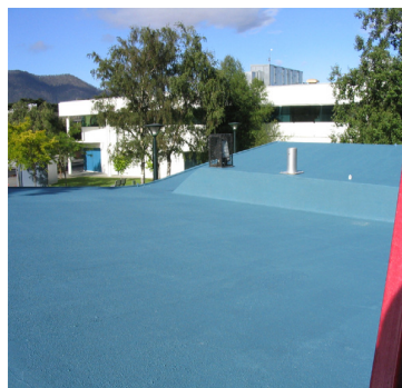
Top Picture: Poly cloth and Watershield A applied to prepared concrete roof
